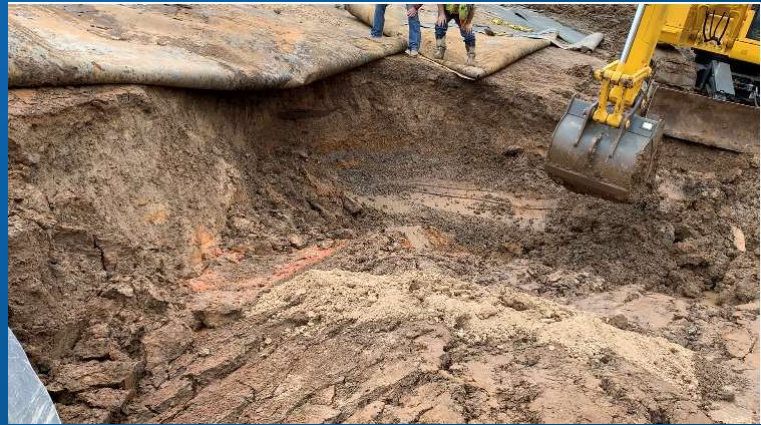
MARCH 2020 – SUSPECT AREA EXCAVATION REVEALAD GROUNDWATER SEEPAGE
