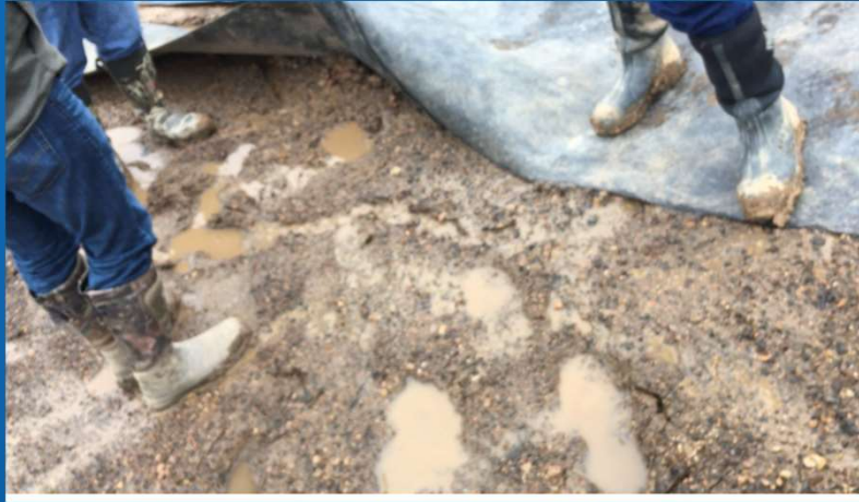
DECEMBER 2019 – SYNTHETIC LINER CUT TO EXPOSE CLAY LINER *** TOO MUCH WET WEATHER TO TELL ***
